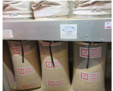
Dust extractor system (Zoff)
