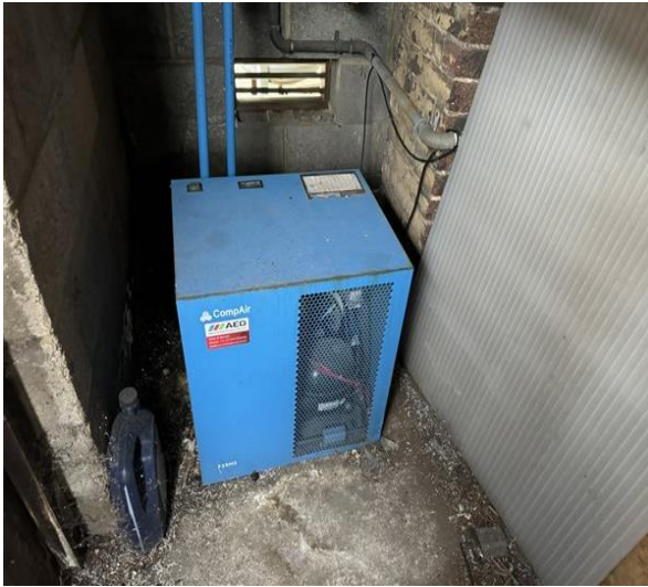
Compair F39 HS refrigerant air dryer
